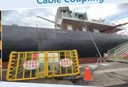
Ship-to-Shore Cable Coupling
